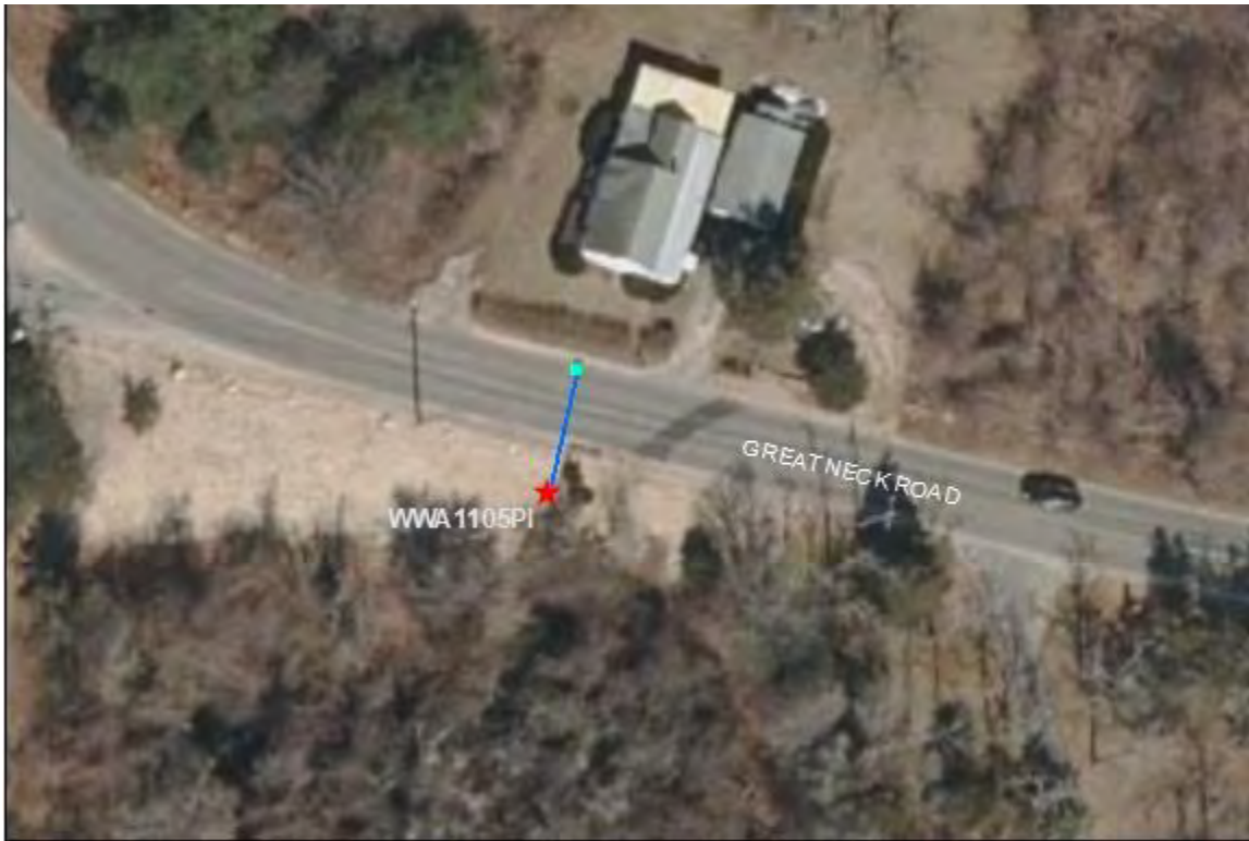
WWA1105PI- Great Neck Road: The catchbasin frame has begun to rot. Preventative maintenance is suggested.
