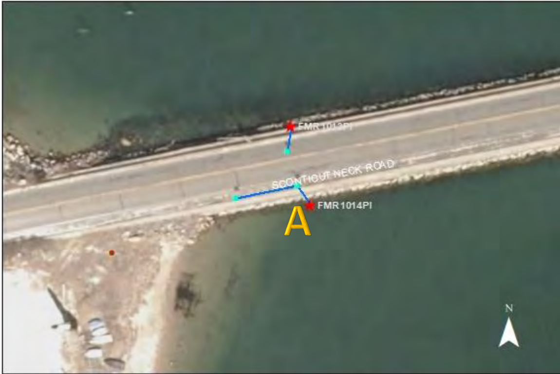
FMR1013PI and FMR1014PI- Scenticut Neck Road: No major issues found. At point A catchbasin is sinking.
