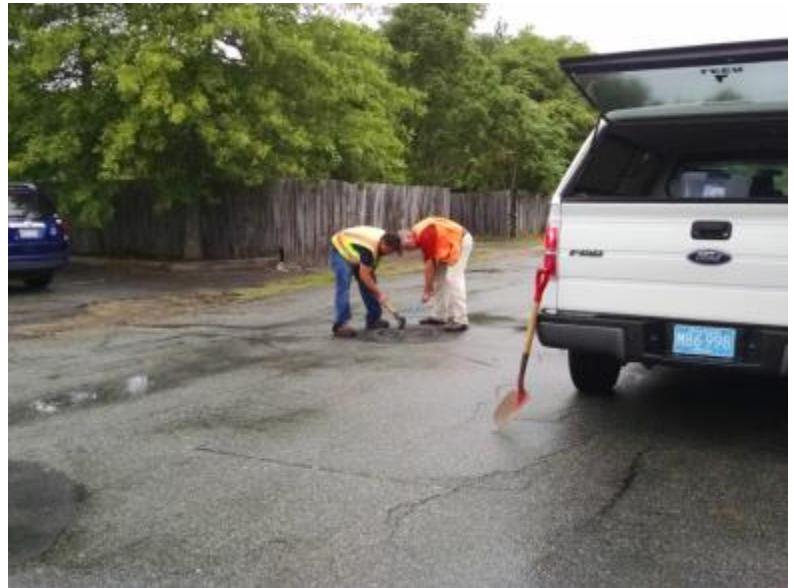
Fig. 8. Manhole covers must be removed to confirm network connections and for sampling.
